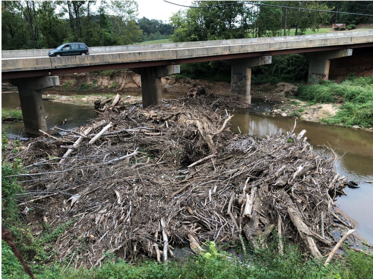
Figure 3 – Debris buildup at the bridge on Power Dam Road in Rocky Mount Va. Photo taken September 18, 2019.
