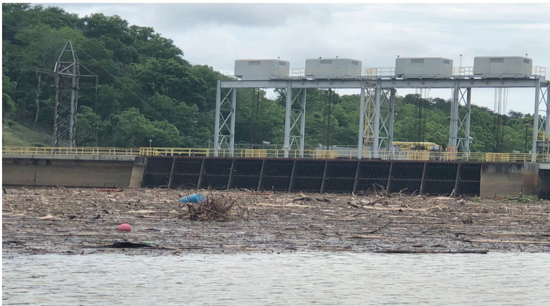
Figure 3.1. Debris collecting in front of Leesville Lake Dam from storm input.
