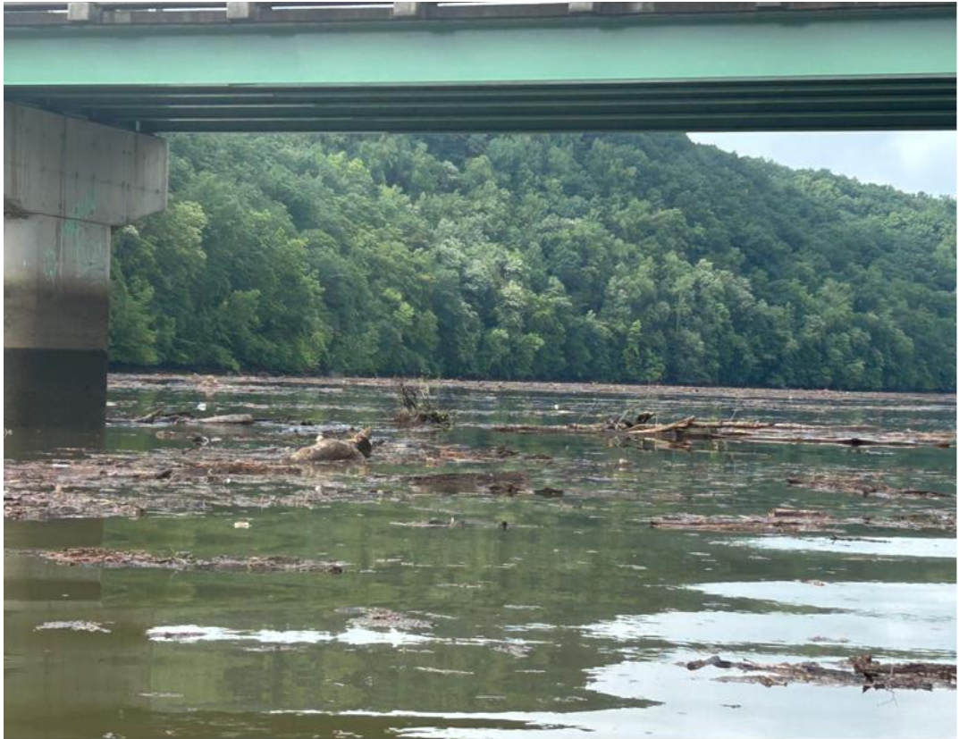
Figure 3.2 – Debris at Toler Bridge June 17 2025 blocking the upper end of reservoir.
